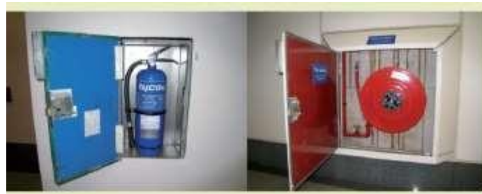
Fig.7. Fire Protection System ( Fire Extinguisger & Hose Reel)
