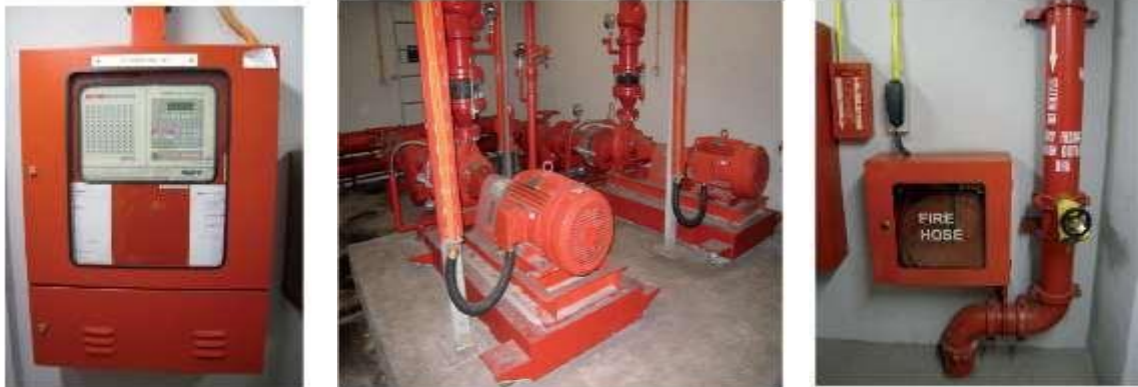
Fig.6. Automatic Detection Supressed System (Fire Alarm Panel, Fire Pump Sprinklers, Dry Main & standby Fire house)
